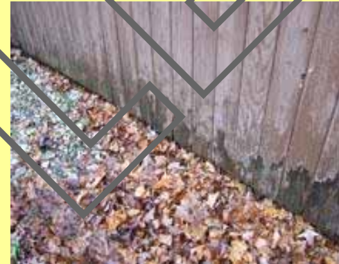
Typical view of the water damaged edges of the siding
