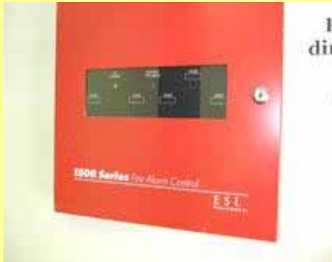
View of the fire alarm panel
