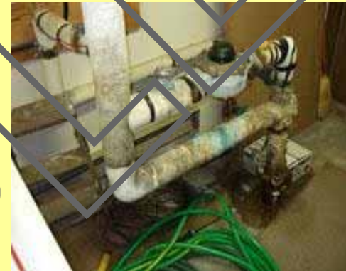
View of the incoming water line
